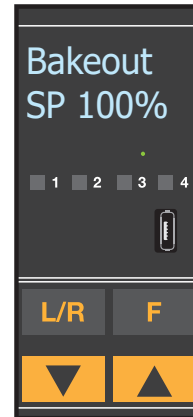
Heater Bakeout Indication
